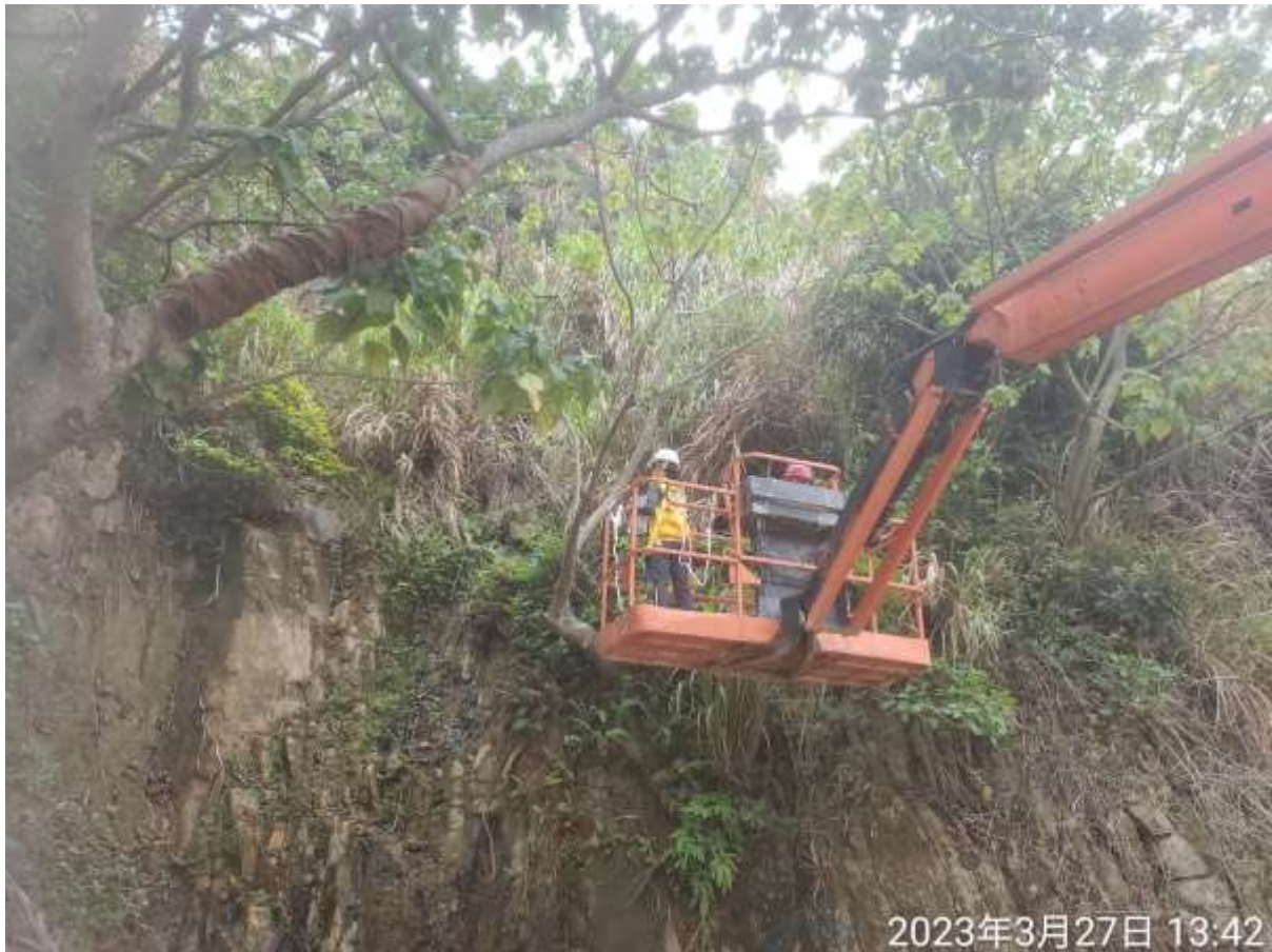
Figure 1 The upper part of the cliff area was assessed by cherry picker.
