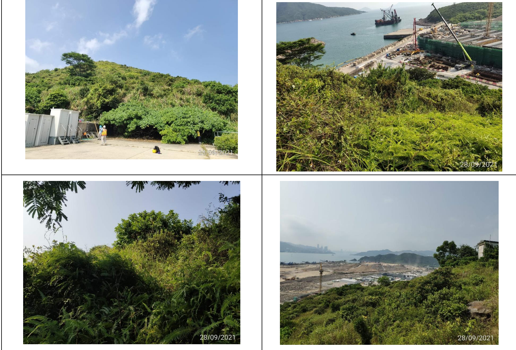
Plate 1. General view and habitat of the proposed Works Site and inspection access of boulder stabilization works.
